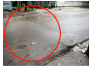
Fig.15 no marking on the speed breakers or speed bumps
