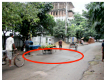
Fig.17 speed bumps can hardly be seen
